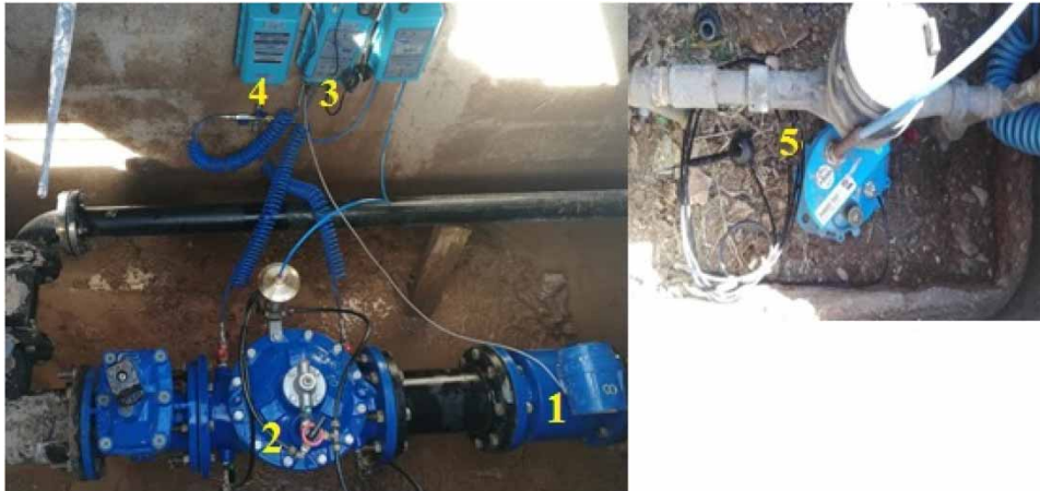
Figure 2 | Real-time instrumentation for pressure management in the city of Chihuahua, México. 1. Electromagnetic flowmeter. 2. Pressure regulating valve (PRV). 3. PRV controller with GPRS communication. 4. Multilog, advanced data logger with integral GPRS telemetry. 5. Multilog, advanced data logger with integral GPRS telemetry at a critical point.
