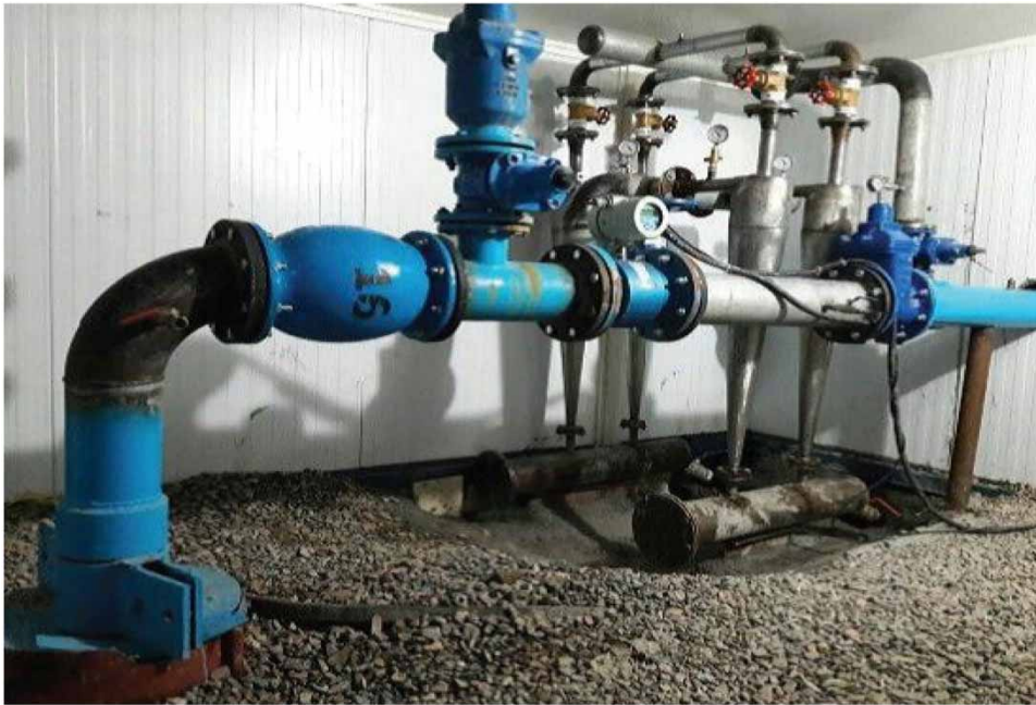
Figure 4 | The optimal medium-scale hydrocyclone installed in a Mashhad well.
