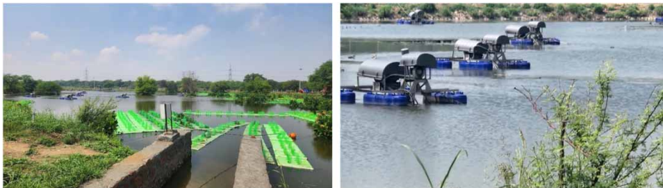
Figure 5 | Floating wetlands and aerators in the artificial water body at Pappankalan STP.
