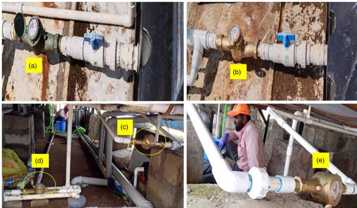
Figure 3 | Water flowmeters installed: (a) male (M) freshwater flowmeter, (b) female (F) freshwater flowmeter, (c) M hand wash & urinal flush flowmeter, (d) M hand wash, urinal flush, and urine flowmeter, and (e) F hand wash flowmeter.
