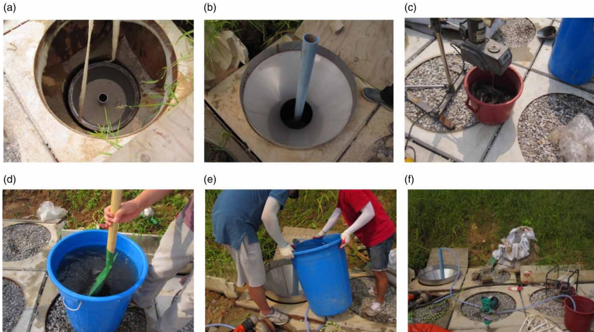
Figure 15 | Field test procedure to evaluate filtration efficiency of sand filter layer: (a) installing sand filter layer into infiltration well, (b) setting floating device and outflow pipe, (c) mixing non-point source pollutants sample with water, (d) preparing artificial urban runoff with non-point source pollutants, (e) pouring artificial urban runoff into infiltration well, and (f) monitoring outflow.
