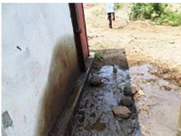
Figure 4 | Stagnant water around borehole.
