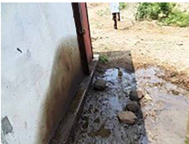
Figure 4 | Stagnant water around borehole.
