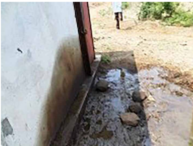
Figure 4 | Stagnant water around borehole.
