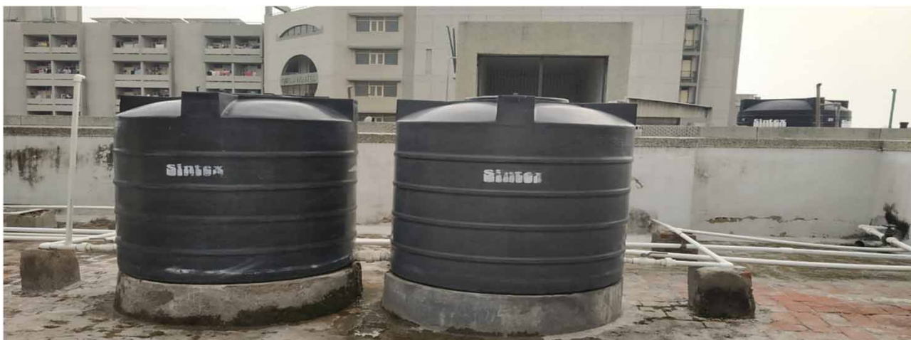
Figure 2 | The water tank system used for data collection.
