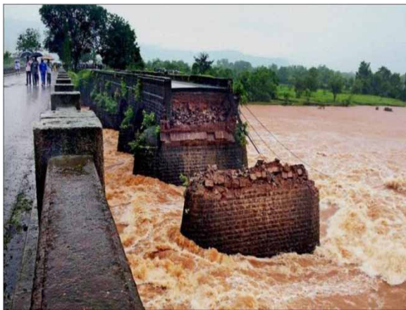
Figure 1 | Collapsed Bridge, Mahad. Source: timesofindia/bridge-collapse-on-goa/liveblog .
