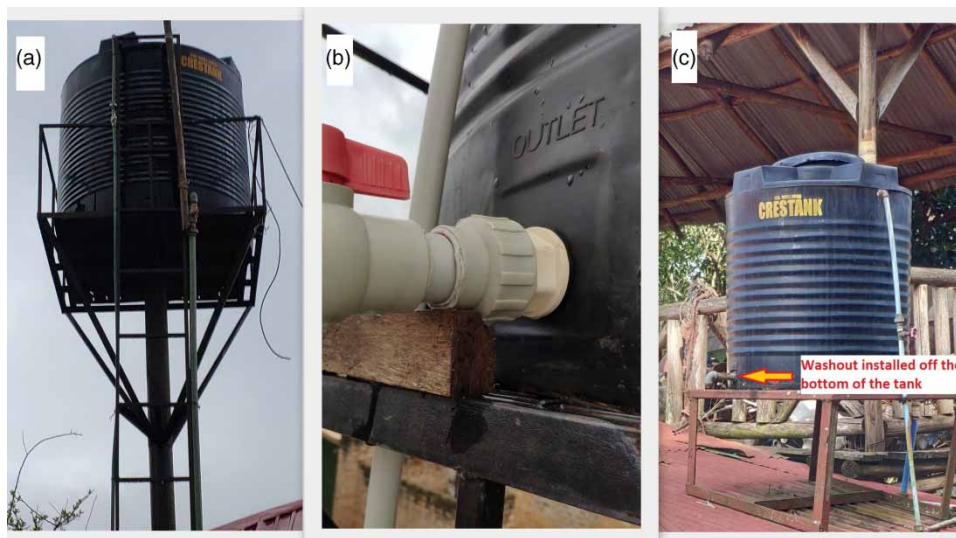
Figure 5 | The manner in which many tanks were installed: (a) a narrow support/tank base; (b) outlet installed off the bottom of the tank; (c) washout installed off the bottom of the tank. Please refer to the online version of this paper to see this figure in colour: http://dx.doi.org/10.2166/ws.2021.411 .
