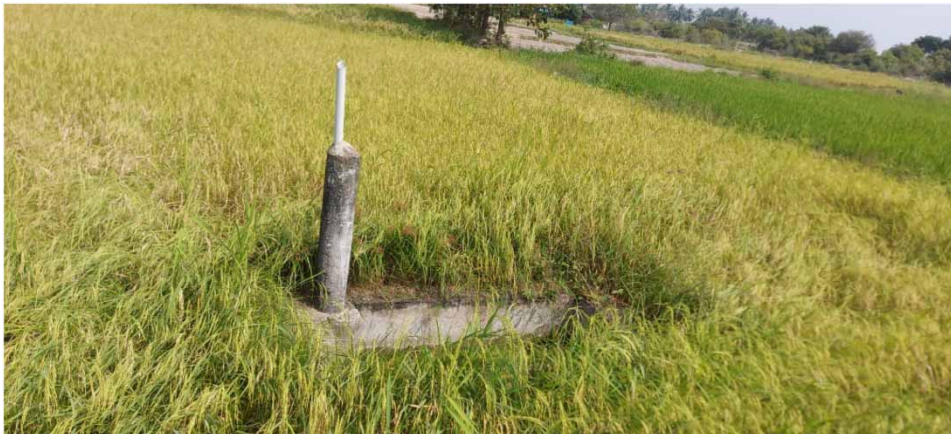
Figure 4 | Air vent pipe in the distribution system in Deevanur tank.
