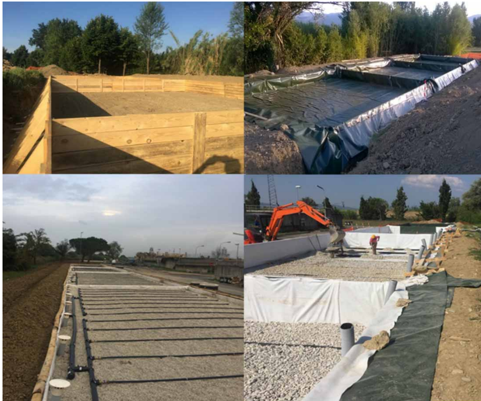
Figure 2 | Different realization steps of the pilot plant. In clockwise order: excavation and forming, laying of geotextile membrane; laying of fine gravel; inflow distribution pipes.
