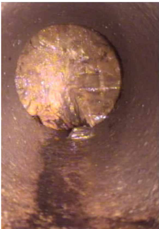
Figure 4 | Hydraulic restriction (blockage) failure along Henry Street, downtown Port of Spain, caused by the solidification of FOG; it caused an SSO, needing an emergency intervention to be cleared (still from CCTV footage WASA).
