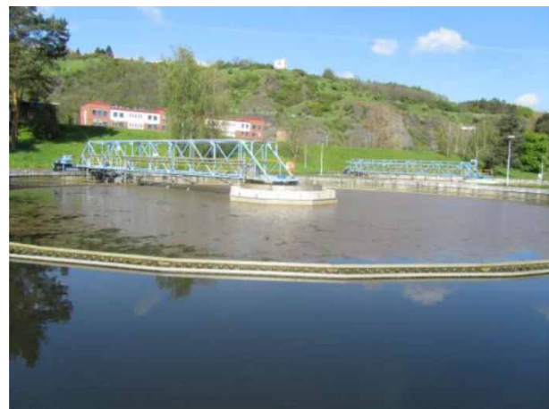
Figure 1 | Secondary clarifier of Prague Central WWTP from the 1960s. Simple energy dissipating well in the center, in-board effluent launder (scum baffles were added later), no surface skimming, sidewall depth 2.5 m.
