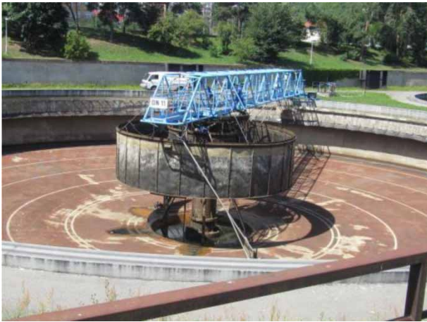
Figure 2 | Secondary clarifier of Prague Central WWTP from 1997. Horizontal flocculation zone, spiral blade sludge scraper, Stamford baffles; sidewall depth 4.4 m.
