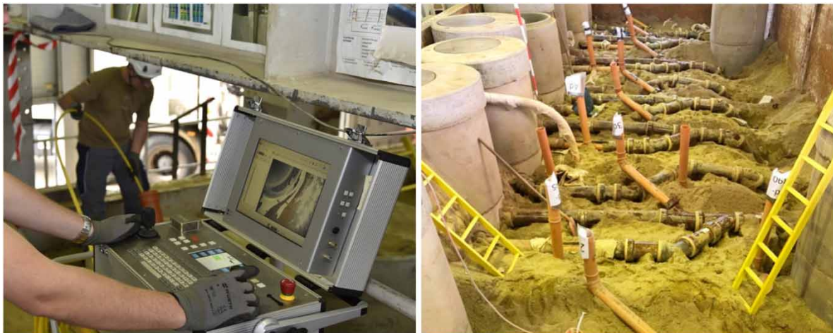
Figure 2 | Carrying out the visual inspection in the covered state under external water pressure (left) and carrying out the internal water pressure tests with inspection from the outside on exposed pipelines (right).
