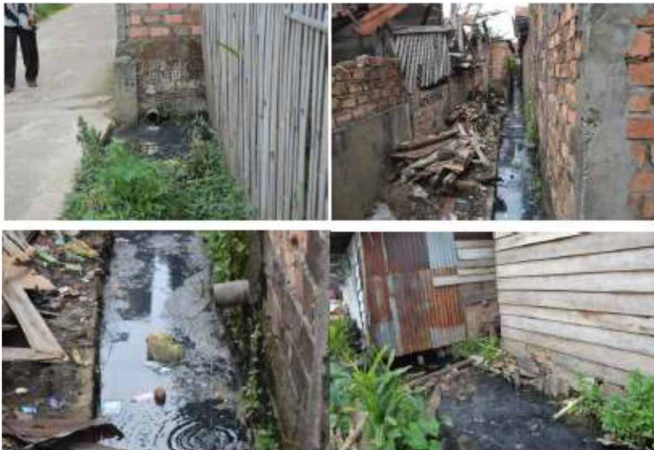
Figure 1 | Combine sewer in Palembang, Indonesia (Rachman 2020).
